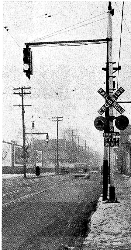
Typical cantilever mounting at Lafayette
